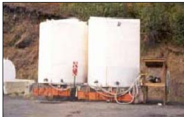
Idaho DOT Chemical Storage Tanks
